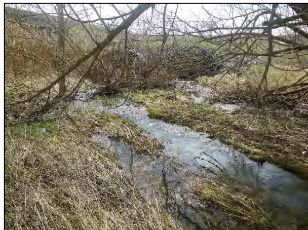
Site 9: Facing east (downstream) at the upstream ends of the 407 ETR culverts (Spring 2019).
