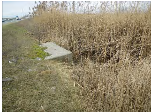
Site 48: Facing west at the upstream end of the culvert conveying flows under Hwy 401 (Spring 2019).
