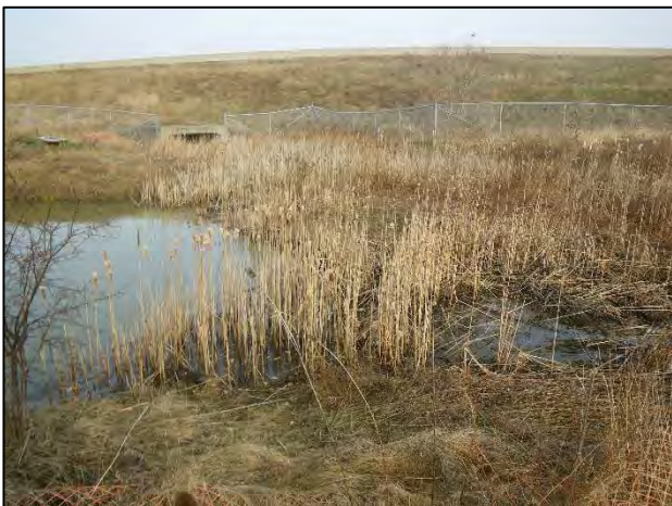
Site 46: Facing north (upstream) at the 407 ETR NBL to Hwy 401 EBL ramp culvert (Spring 2019).
