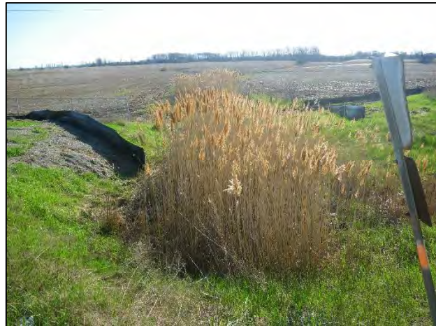
Site 36: Facing east (downstream) from the downstream end of the Trafalgar Road culvert in the runningway and station location (Spring 2019).
