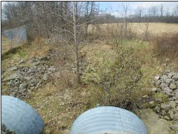
Site 8: Facing west (upstream) from the upstream end of 407 ETR culvert (Spring 2019).
