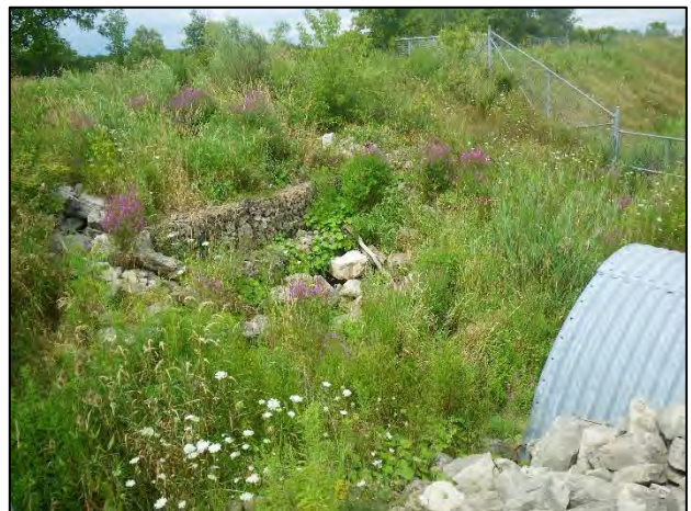
Site 6: Facing northwest (upstream) at the upstream end of the 407 ETR culvert. Note gabion basket barrier to fish passage (Summer 2019).
