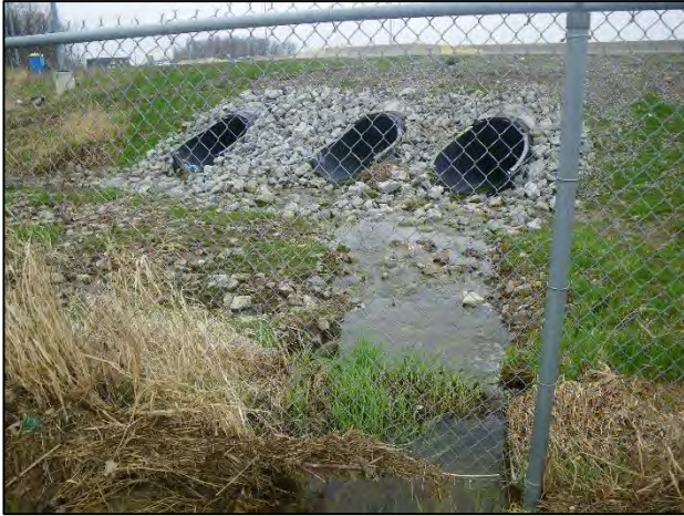
Site 18: Facing east (downstream) at the upstream end of the 407 ETR culverts (Spring 2019).
