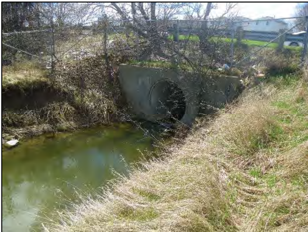
Site 4: Facing south (upstream) at downstream end of pipe outlet at Guelph Line (Spring 2019).
