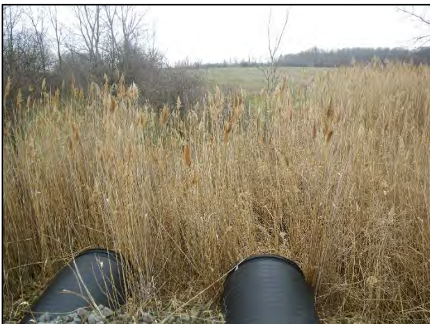
Site 23: Facing south (downstream) from the 407 ETR EBL lane offramp culverts (Spring 2019).
